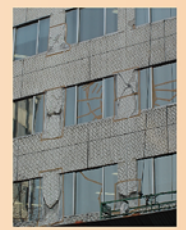
Damaged exterior walls and broken windows (West of Fukuoka Prefecture Earthquake)
